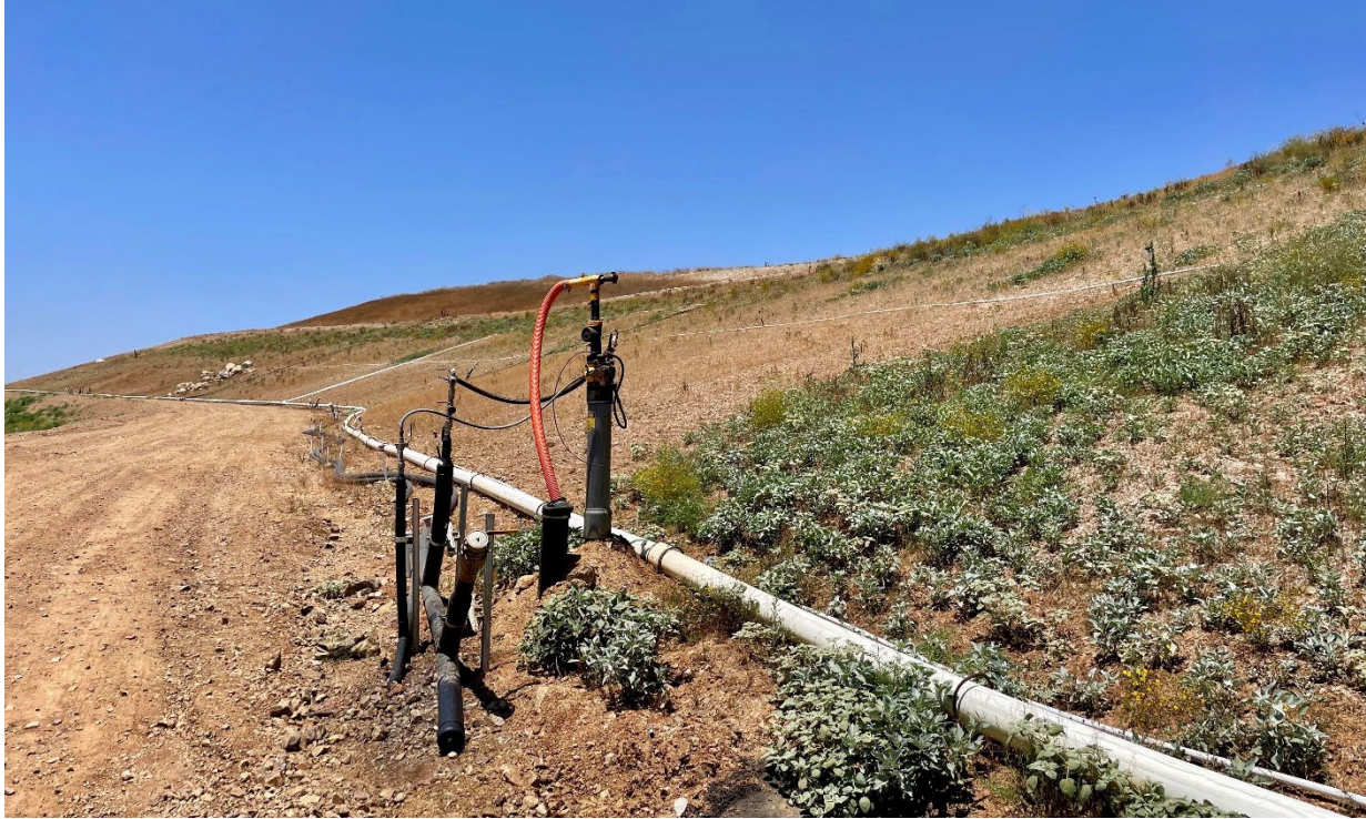
Photograph 17. Phase D1 irrigation system and a monitoring well, June 22, 2023.
